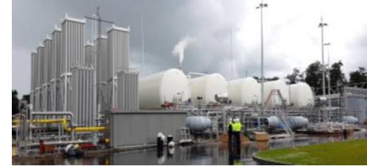
LNG reloading and bunkering station in Klaipeda
