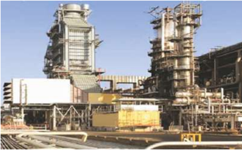
ExxonMobil Antwerp CHP Belgium (125 MW)
